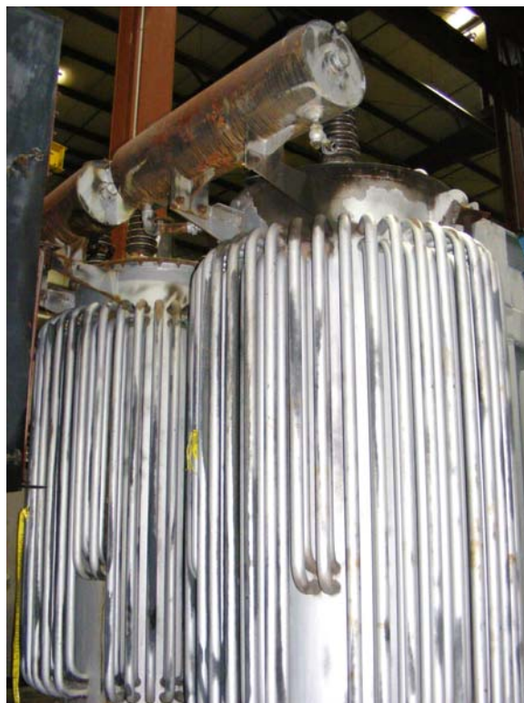
Photograph of GE Transformers contaminated with DBDS FIGURE 11
